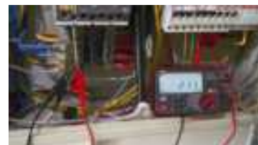
Automatic Voltage Measurement
